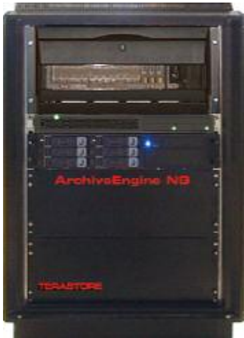
ArchiveEngine® NG (NAS-Filer, RAID, Tape-Library) im 19" Rack
